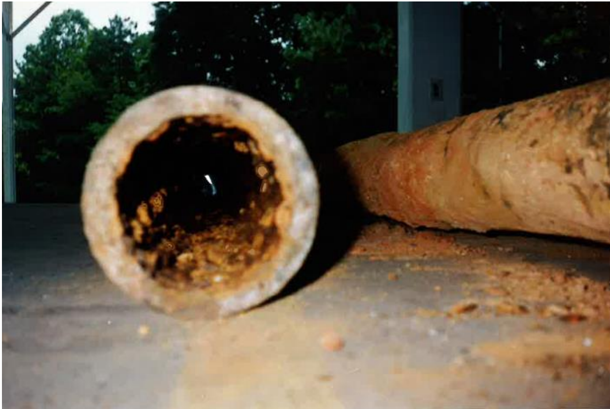
Image 1: Heavily corroded pipe previously treated with zinc ortho phosphate
