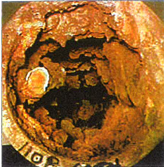
Corroded pipes comprise about 40 percent of the District's distribution system.
